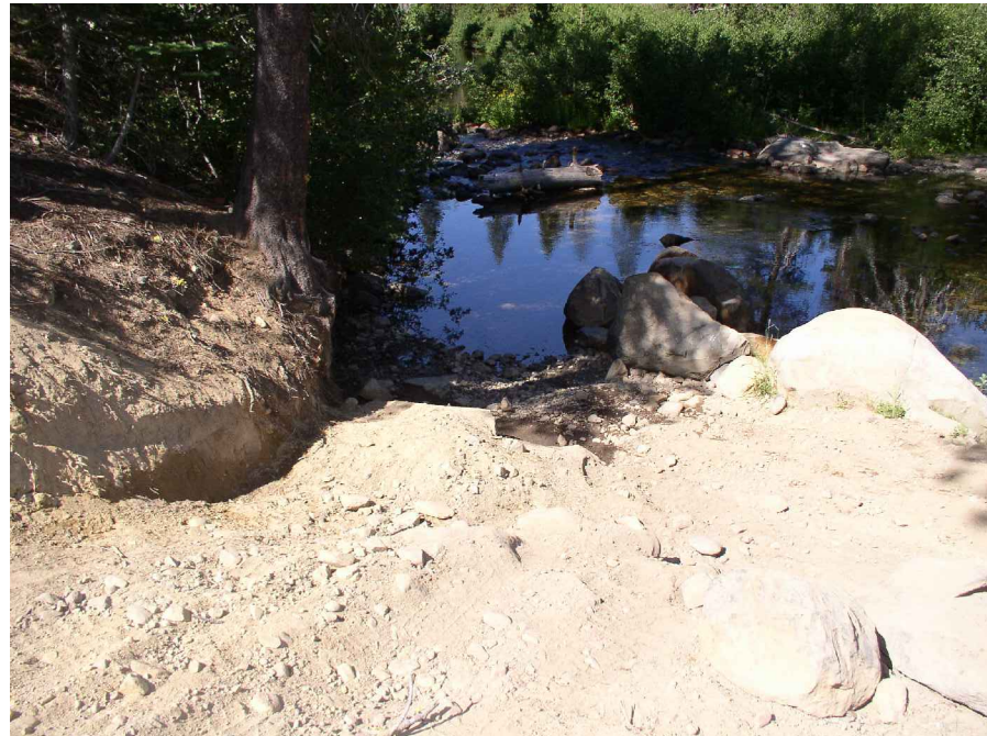
PHOTO K (Aug 2006) View of existing low water crossing from Abutment 2 location.
