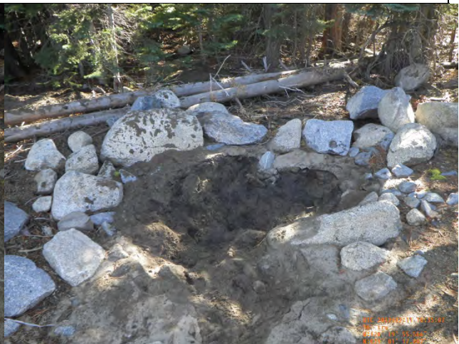
Rock Energy Dissipater LL Station 148+75.49 RT Post-Clean
