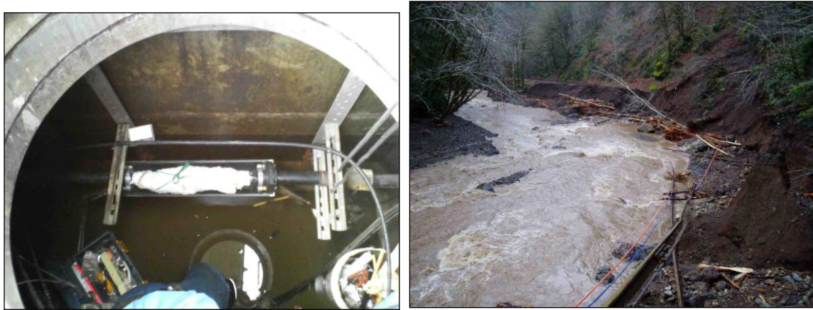
Figure 40. Damage to fiber optic cables: flooding degraded transmission when water leaked into a splice (left); ground failure damaged a cable laid along a railbed that washed out (right).
