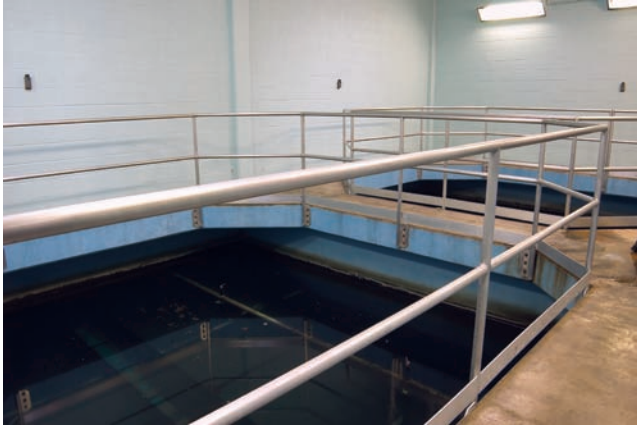
Water System Filtration Tank
