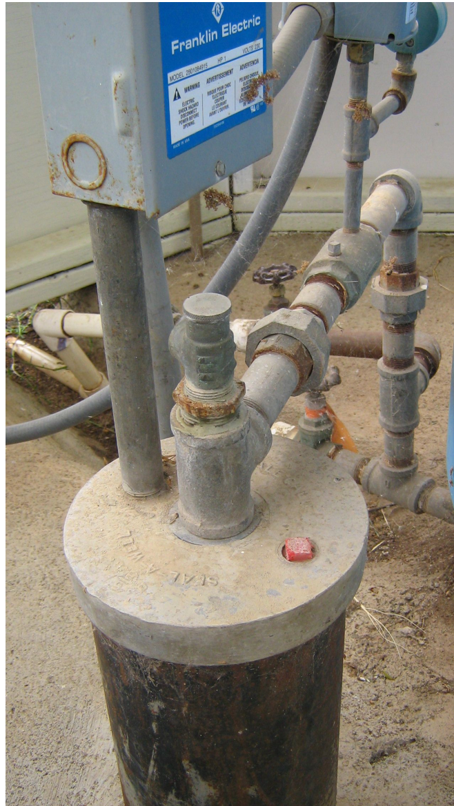
Photo: A domestic well showing the well casing, cover, and conveyance system. The well is located inside a shed with a concrete floor.
