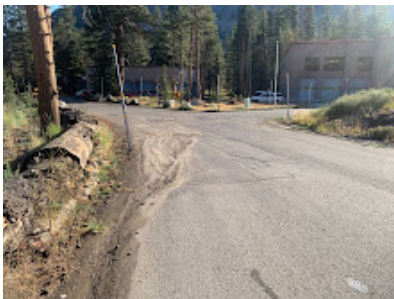
Loop Road Drainage Issue 9.6.22 #3.jpg 1543K
