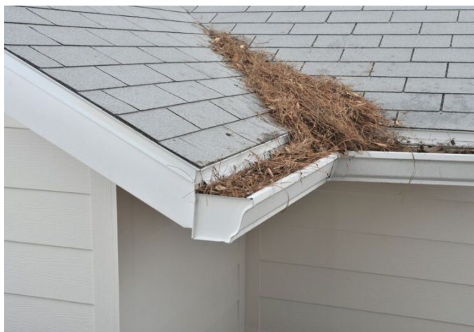
Figure 69. Roof with an accumulation of pine needles at the roof valley, creating a potential fuel bed for ember ignition.
