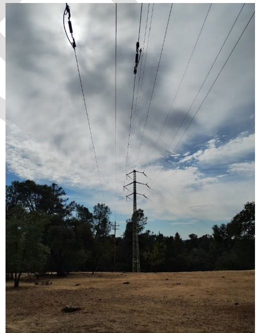
Figure 86. Appropriate clearance around critical communication infrastructure is essential for agency and public communication and messaging during incidents, particularly as this equipment is typically located in high fire hazard topographies.
