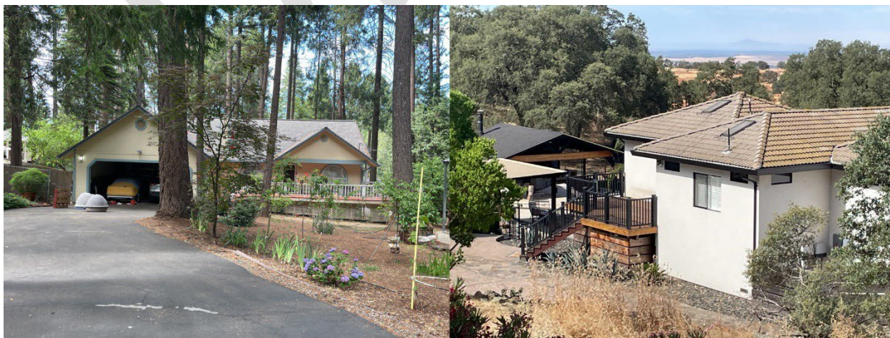
Figure 71. Crawlspace under decking screened in with combustible materials.
