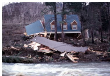
Photo 2: Cabins damaged and destroyed by the massive Mill Creek landslide that occurred on January 24, 1997. USGS Photo by Mark Reid, USGS/Menlo Park, 1997
